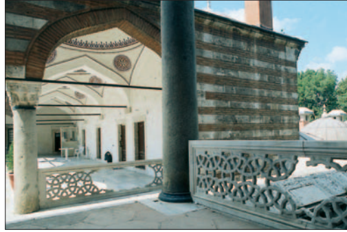
Illustration 11. Zal Mahmud Pasha Mosque, the condition of the west wall of the külliye suffering from traffic. (Photo: Aras Neftçi)
